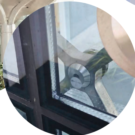
Mövenpick Hotel and Convention Centre KLIA in Sepang, Selangor uses GP Glass' double glazing glass panels unit with holes.
